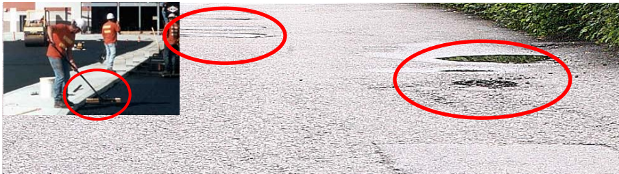
Hand made pavement. Pavement with irregularities and holes.
